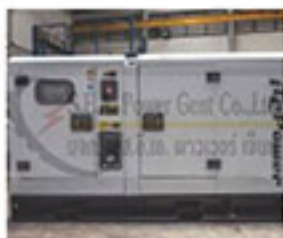
ITC Power DG 22 KSEm 22 kVA
