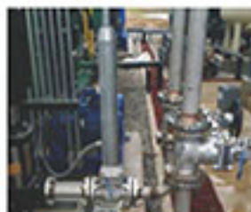
Industrial Piping Work
