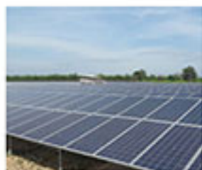
Solar Cell Supporting Structure
