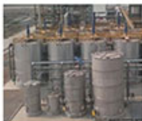
Silo Storage Tank
