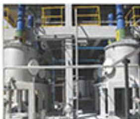
Industrial Vacuum System
