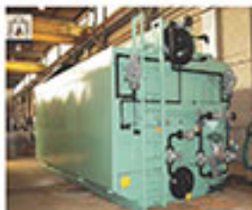
Cleaver Brooks Water Tube Boiler
