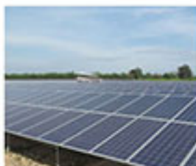
Solar Cell Supporting Structure
