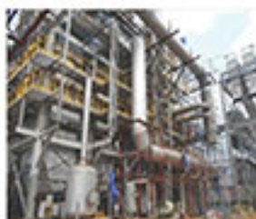
Structural Steel Pipe Rack
