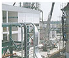
Structure Pipe Rack
