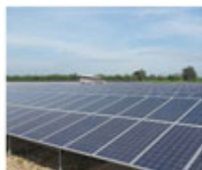
Solar Cell Supporting Structure
