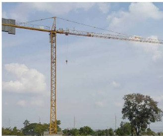
Tower Crane Potain ម៉ាក 85 B
